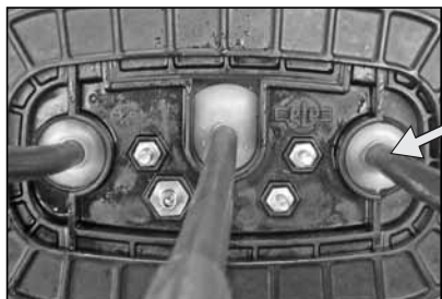
Leak occurring at the cable entry of the grommet
